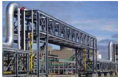
Pipe Support Structures
