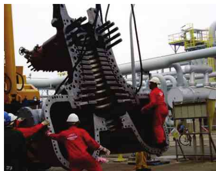
Part of a Steam Turbine
